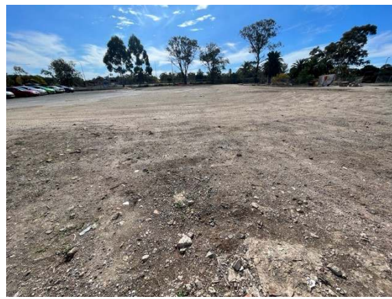
Photo 4: Surface inside the site compound required further stabilisation to reduce risk of dust and tracking
