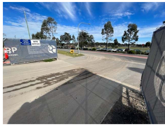
Photo 5: Tracking observed from the site compound onto De Clambe Drive
